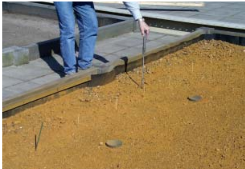
Figure 7: Use of the Dutch Cone Reflectometer on one of the test lanes
