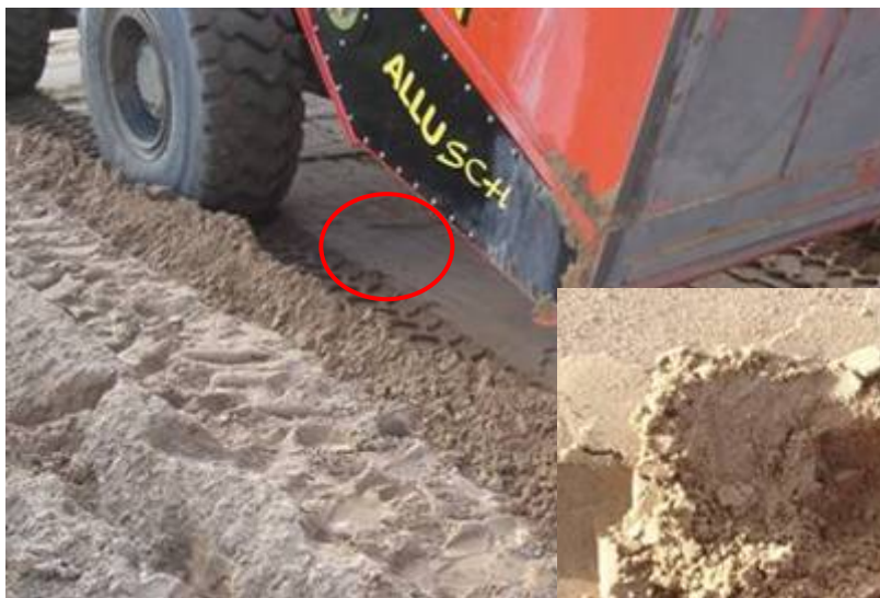
The potential risk of missed mines is clearly visible here.
