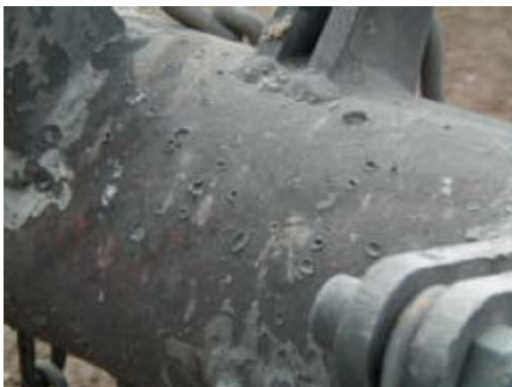
The picture shows splinter damages to the flail pipe
