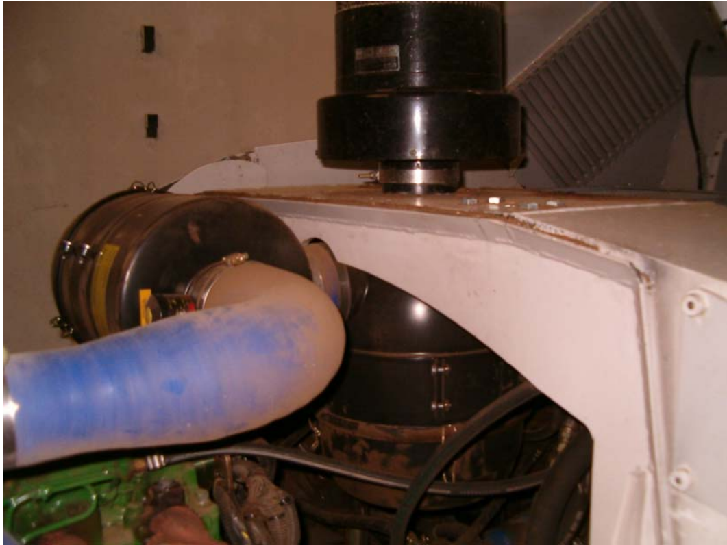
Figure 2-2 Three-stage filtration unit
